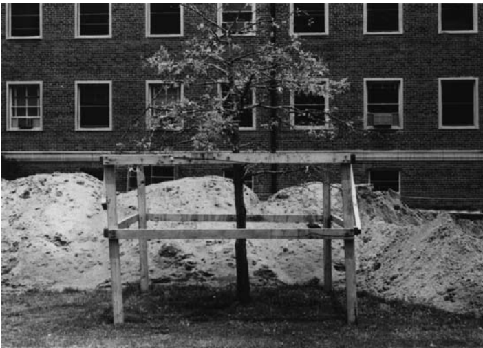
Figure 1. This fence is not sufficiently large to provide much protection for roots of this young tree. The stem is about eight inches in diameter near the soil line and lower branches were recently cut off so they did not overhang the fence. For this tree to have a good chance of survival the protection area should have been at least doubled.
