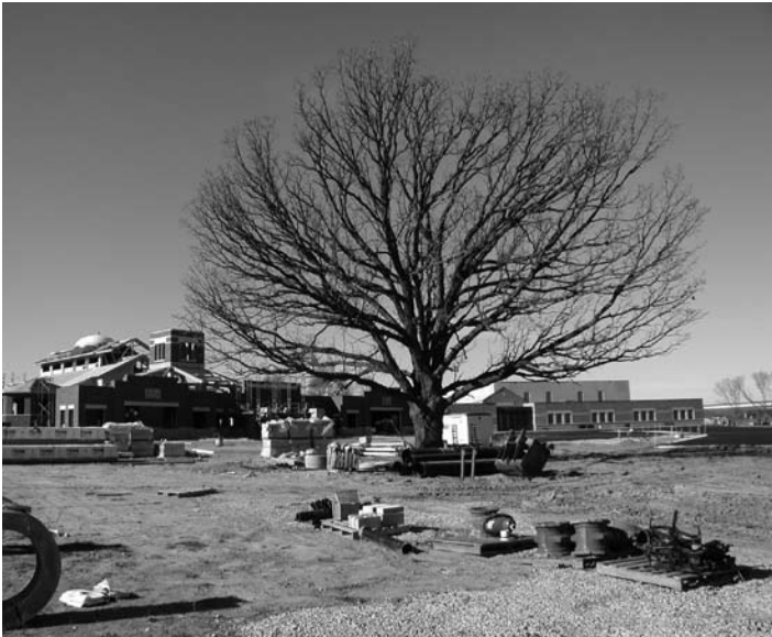
Figure 2. The site was a church-school combination. All vegetation was removed and grading done, except, for one large, beautiful bur oak that was initially left undisturbed. Access to the site and loading and storage of materials was from the lower left area of the photo, including entrance and exit of cement trucks.
